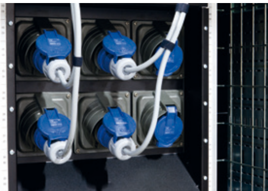
Power distribution rack
