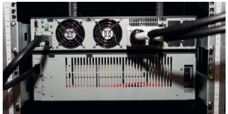
Power distribution rack: UPS systems
