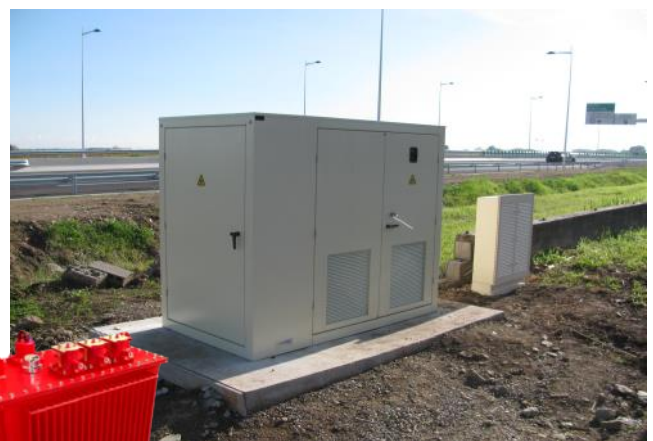
Outdoor substation PTS95 with 50 kVA watertight transformer
