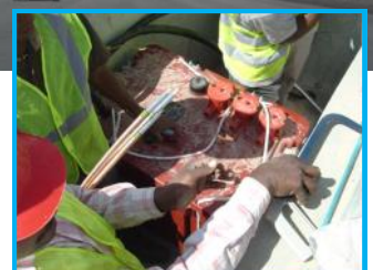
Pit with TER transformer 32 kVA
