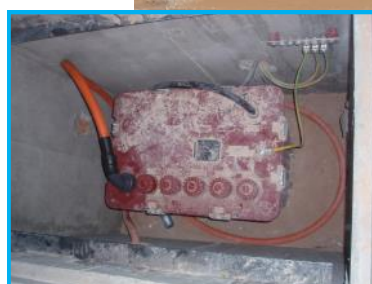
TER TT in a pit
