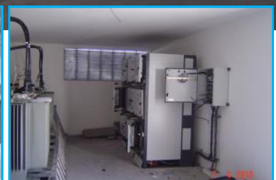
Substation with 5500 V switchboard
