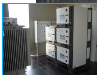
Substation equipped with 6,6 kV switchboard
